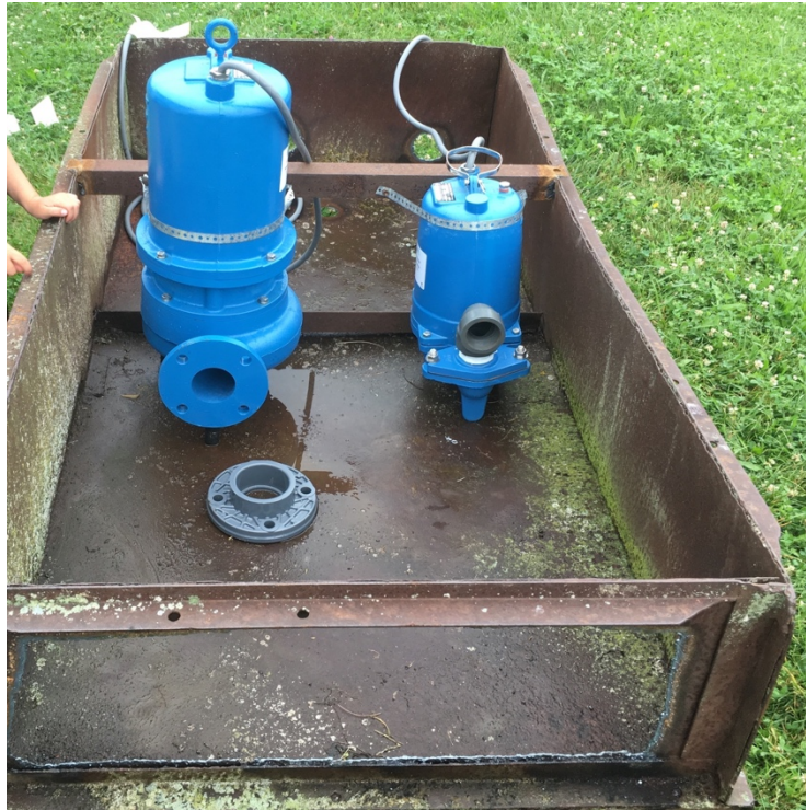
Figure 6. Submersible pumps and metal stand that were placed in the secondary waste treatment pond. The larger pump moved 1,249 lpm (330 gpm) and the smaller pump 984 lpm (260 gpm). A 100% water exchange occurred approximately every 21 hrs 50 min.
