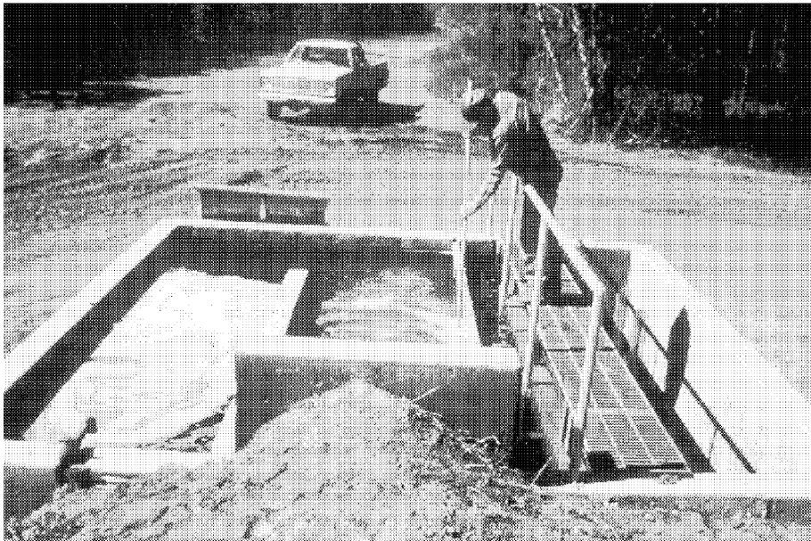
Figure 6. An outside catch basin at the Garrison Dam National Fish Hatchery, Riverdale, North Dakota. A schematic design for this catch basin is given in the case study by Call (1996).
